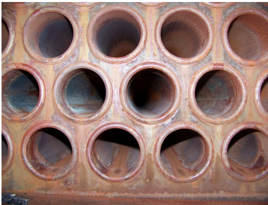
Fire Side of Fire Tubes
