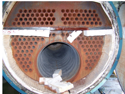
Fire Section of Boiler
