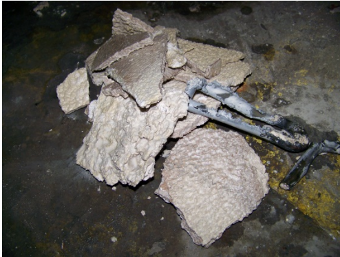
Boiler #1: Scale from Bottom Hand Hole
