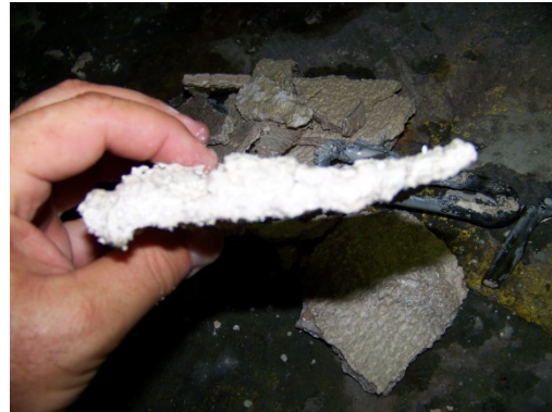
Boiler #1: 1/2" Thick Scale from Bottom Hand Hole
